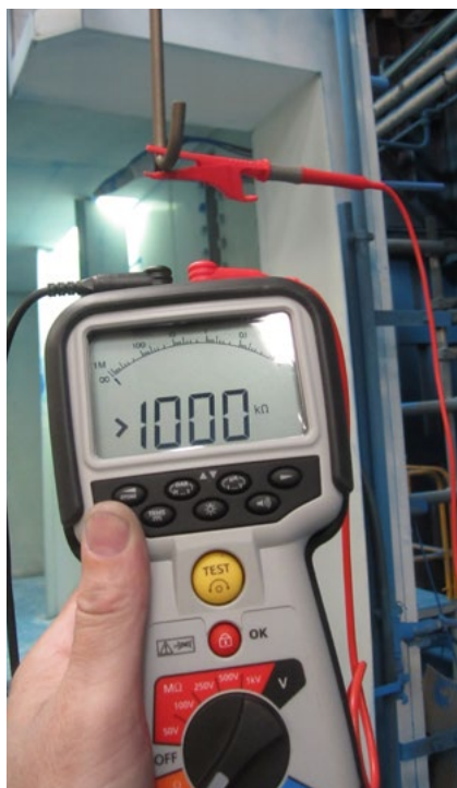
Ground continuity measures under 500V.
